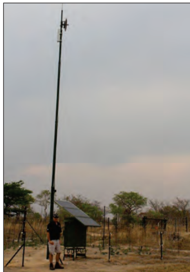
Solar installation with wireless link to base camp
